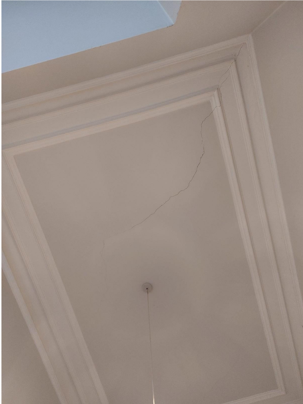
Photo 2: Example of crack to internal ceiling finishes
