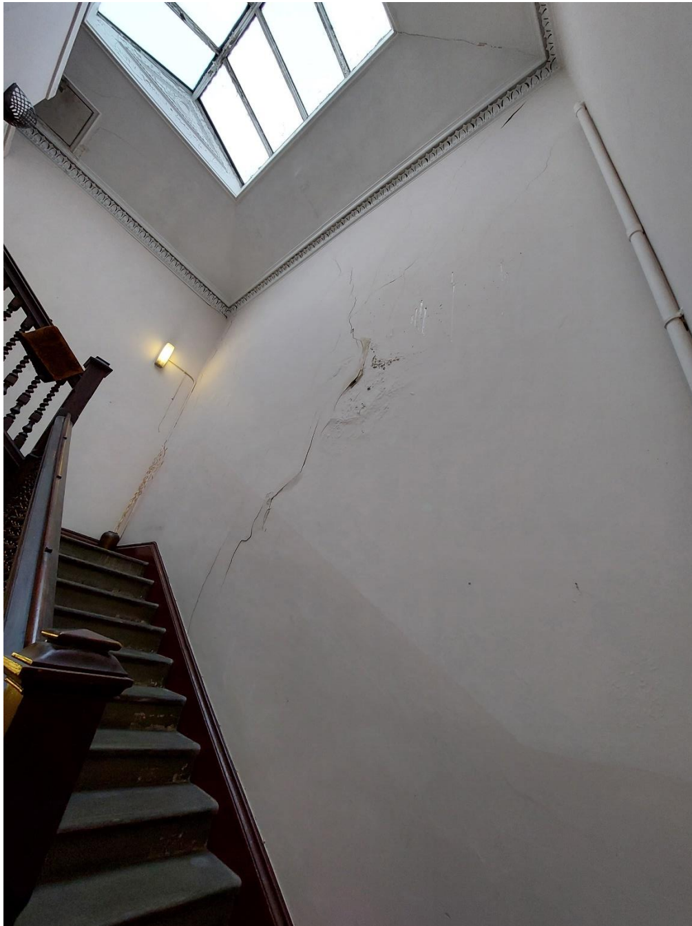
Photo 1: Main cracking to party wall
