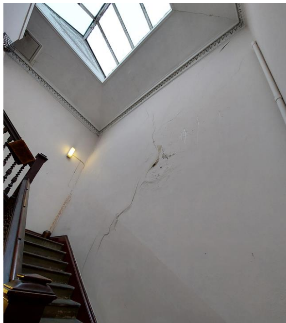
Figure 1: Site Photo of cracking to party wall at 2 nd floor level
