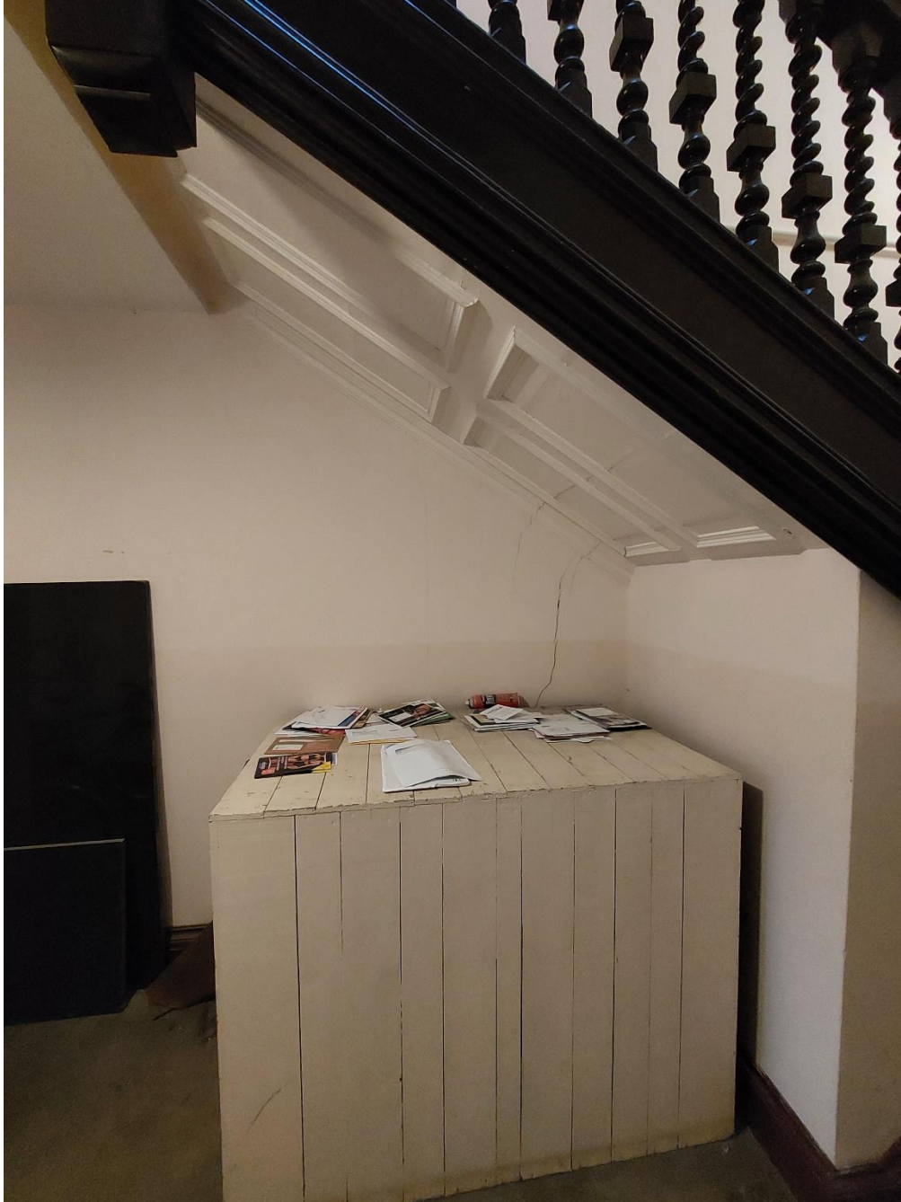
Photo 3: Minor cracking to ground floor party wall and cantilever stair
