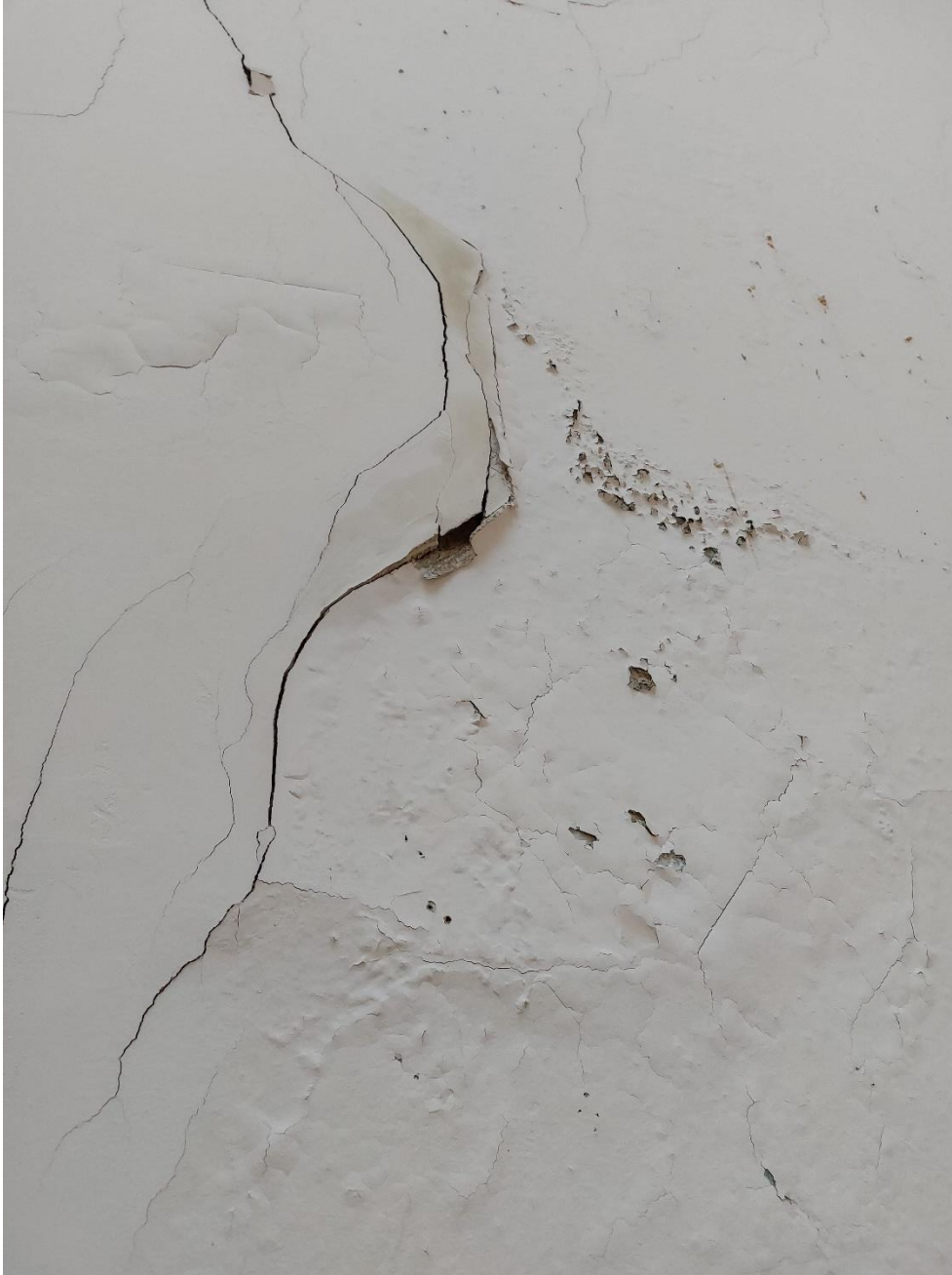
Photo 5: Clear signs of moisture/damp to worst section of cracking
