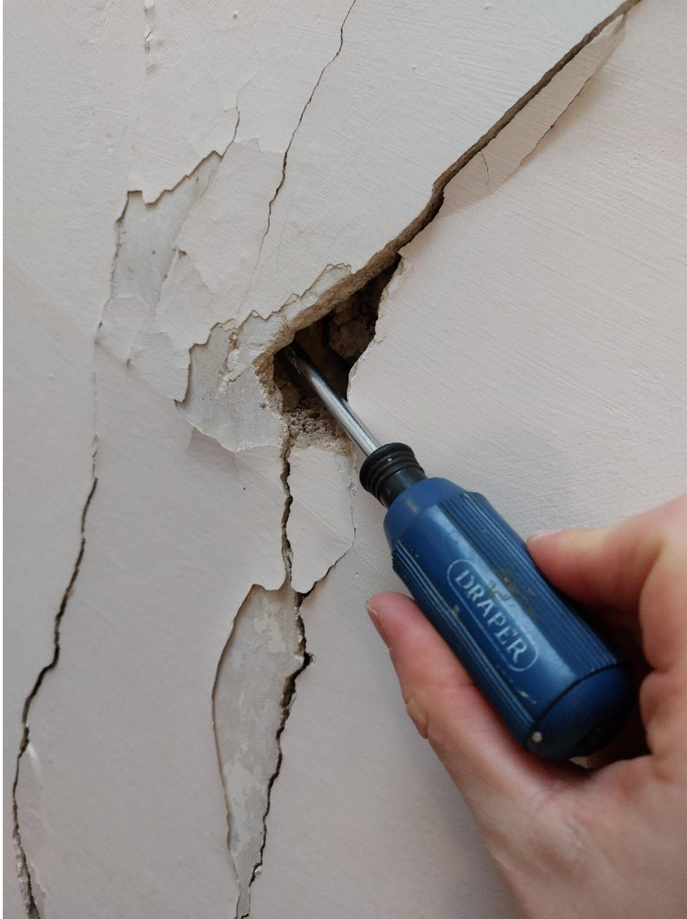
Photo 6: Plaster has delaminated from masonry behind locally at the bulge in the crack. Cracking did not appear to extend into masonry behind on probing
